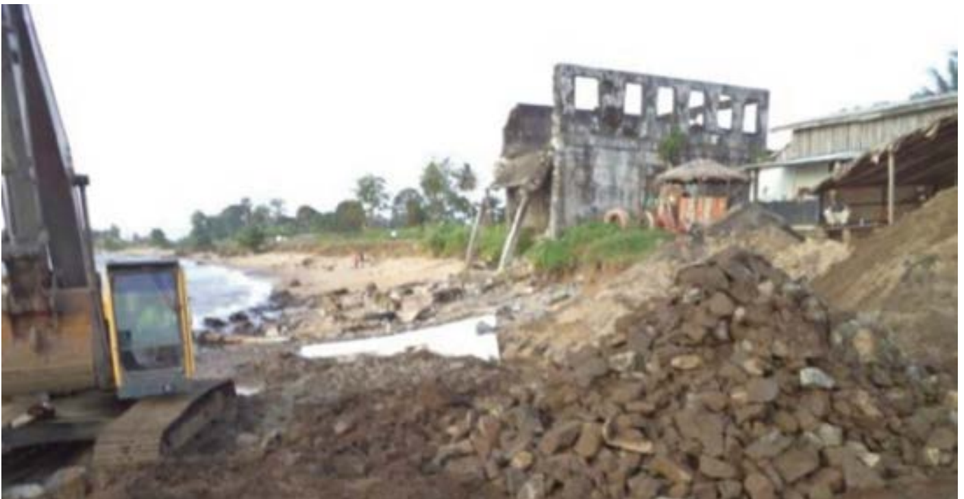
Implementation of the first matte GeoTextile section (white color in the image) below the construction to protect the concrete structure in Buchana
