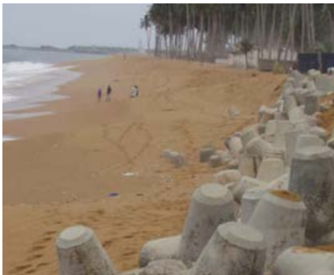
Breakwater lines facing a protective wall in front of Coco Beach. Port-Bouet, Abidjan (October 2003). Source: SDLAO's detailed case study report, Côte d'Ivoire).
