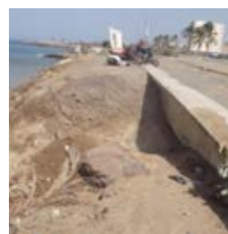
The erosion of coastal road formations is largely dependent on storm water management (Source: MOLOA country branch of Senegal)
