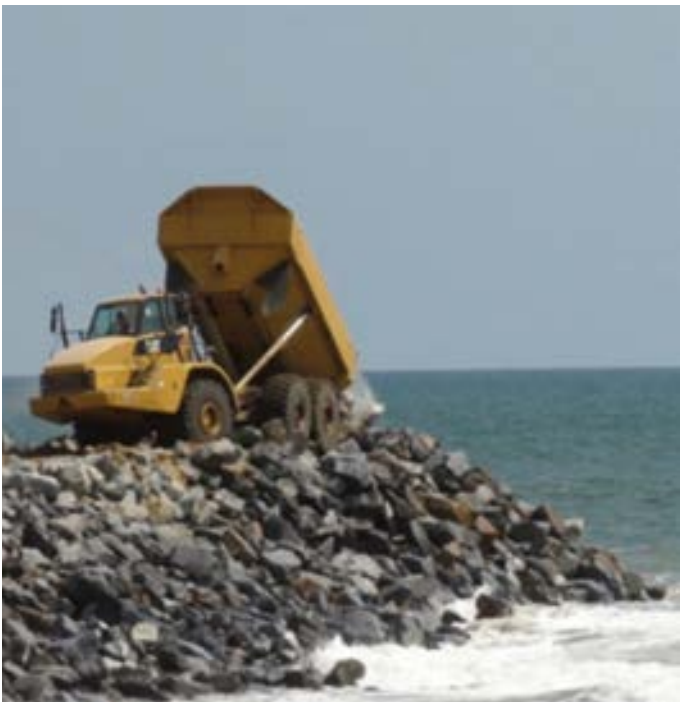
Development of the spurs system west of the port of Cotonou (source: MOLOA's country office in Benin)
