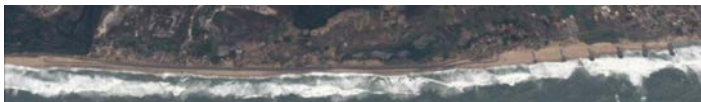
Protection works building of the coastal road between Salo and Angola (2010-2013) on the left bank of the Volta
