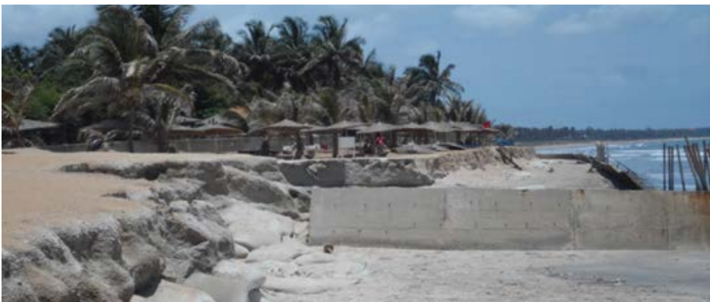
Despite major beach re-sanding operations a few years ago, erosion is apparent and significant in front of the big hotels of Serrekunda. The Gambian authorities are closely monitoring the situation.
