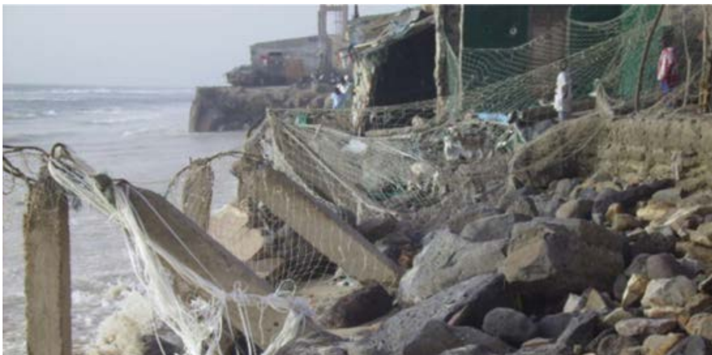
Collapse of the protective wall in Guet Ndar (built in 1910 and which is has already crumbled in a major part). Picture Marsh 2010, Leïdi (source; case study).
