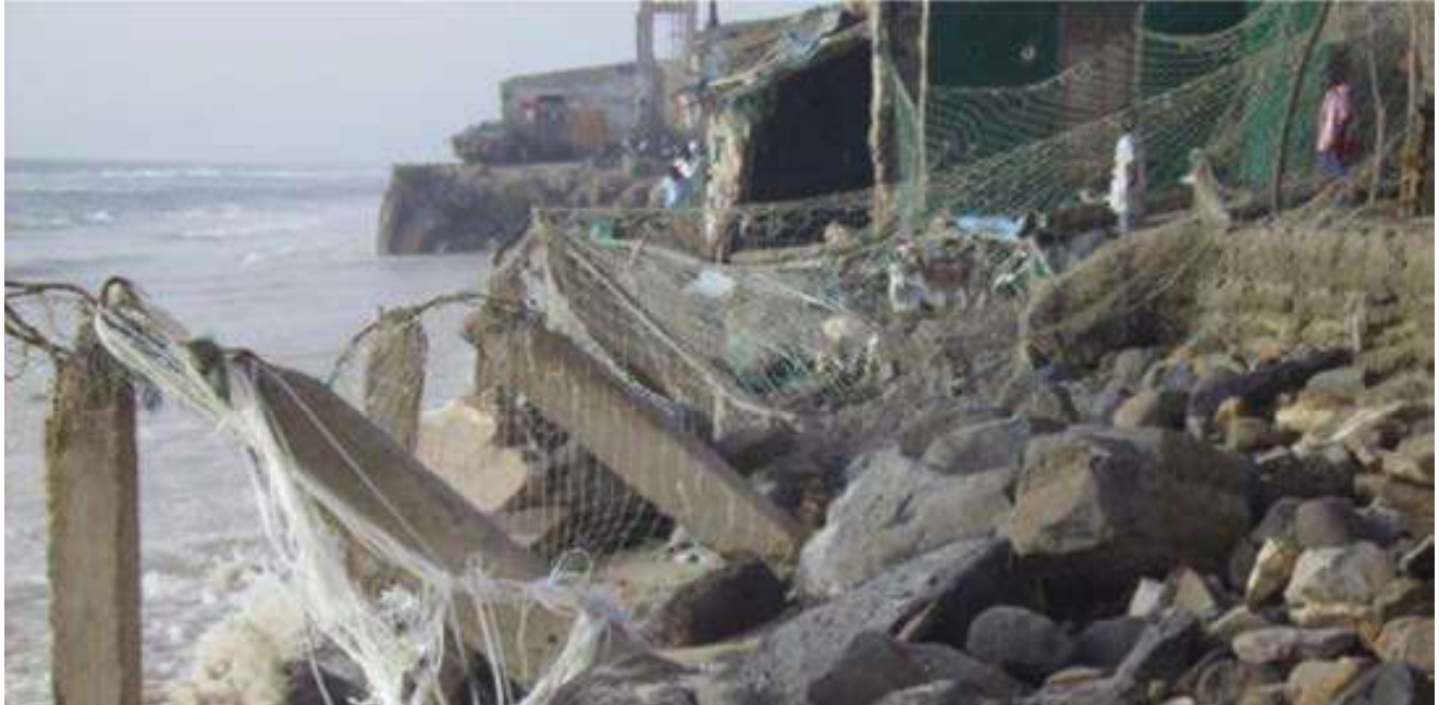
Collapse of the protective wall in Guet Ndar (built in 1910 and which is has already crumbled in a major part). Picture Marsh 2010, Leidi (source; case study).
