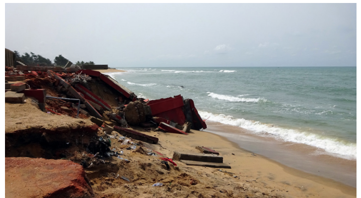
PHOTO 1 Erosion has destroyed houses in Baguida, Togo
